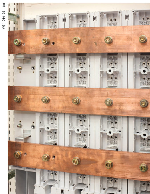
ISFL250 (direct connection on 185 mm 2 busbar).
