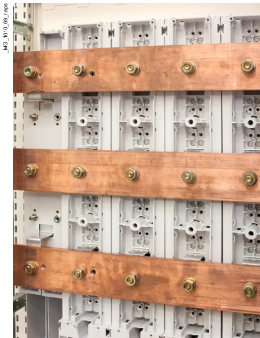
ISFL 160 (direct connection to the busbars).
